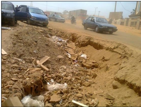
Figure 2. Taki Road and the Drainage System before the road dualization (Improper planning)
