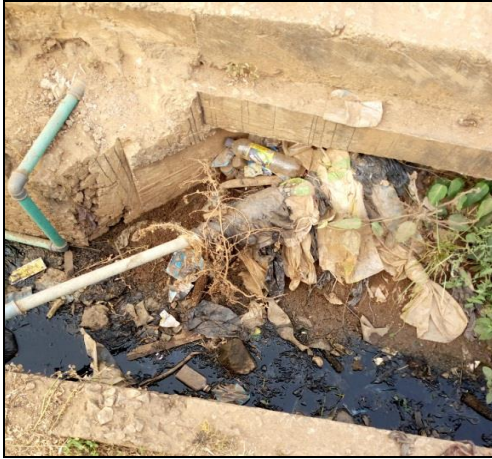
Figure 6. Storm Flow Obstruction by Utility Lines
