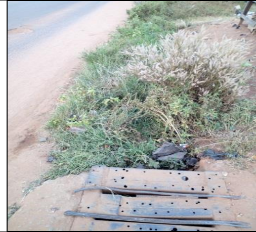
Figure 7. Drainage Channel Overgrown by Vegetation
